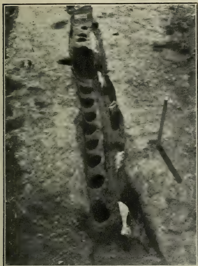
a. Horizontal mold between vertical molds and line of stones on outside wall of trench. Structure No. 1, Site No. 5.
